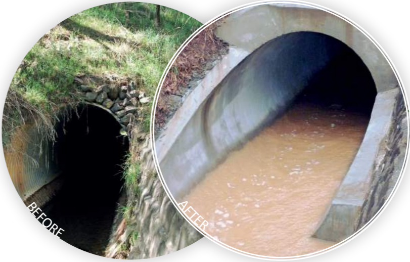
2300mm diameter Corrugated Steel Culvert Location Hume Highway, Broadford, VIC Client VicRoads
