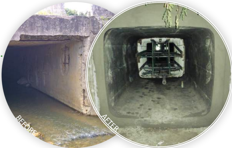
2400 x 2100mm Concrete Box Culvert Location Colliery Access Road, Kemira Valley, NSW Client BHP Billiton Coal Contract Services
